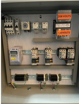
Control Panel Interior
